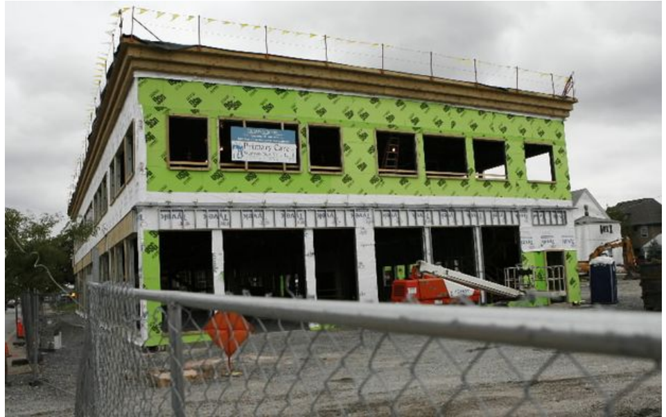
The new mixed-use building, which will include retail and office space, sits at the former Kane Doyle Jeep site in Kenmore. (James P. McCoy, The Buffalo News)
